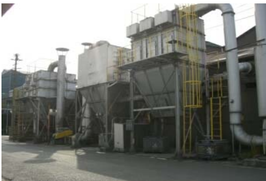
Example of installation of a large dust collector
