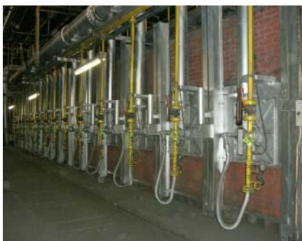
Tunnel type furnaces
