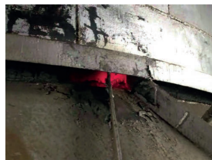
Fig. 17 Photo of steel shell red-hot part.
