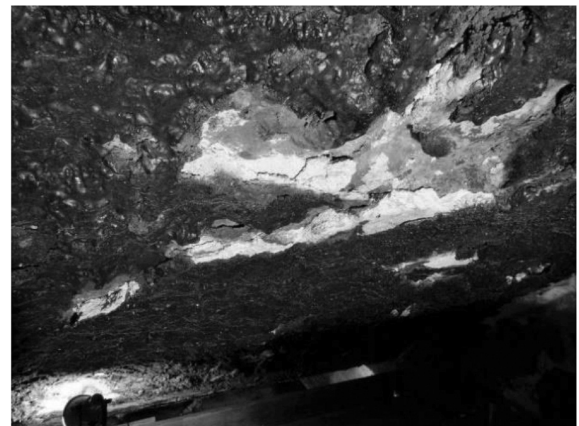
Fig. 12 Photograph showing surface condition of gunned body experiencing 6 months incinerator operation.
