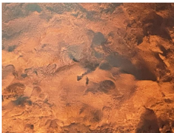
Figure 13 Appearance of refractory peeling
