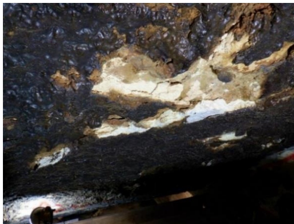
Figure 12 Appearance of Material A after six months of furnace operation
