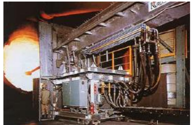
Fig. 11 Large thermal spraying machine for converter.
