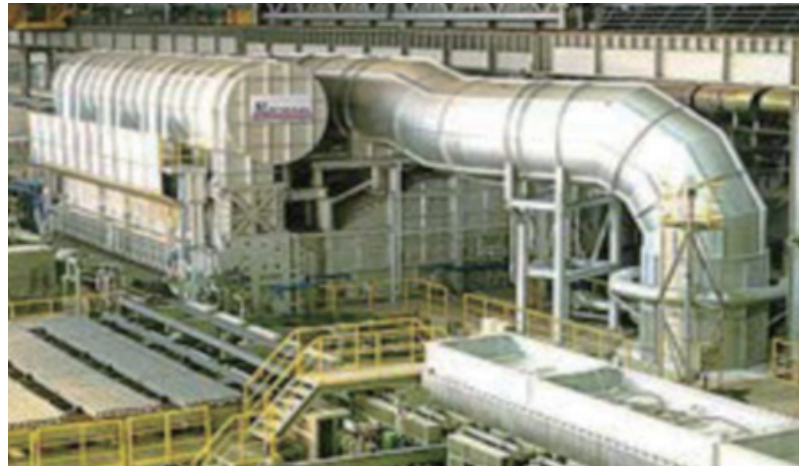
Photo 5-4 Energy-saving reheating furnace
