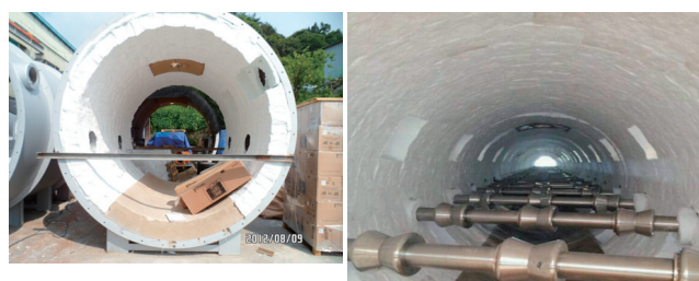
Fig. 4 Installation in heat treatment furnace -2
