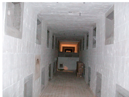
Fig. 3 Installation in heat treatment furnace -1
