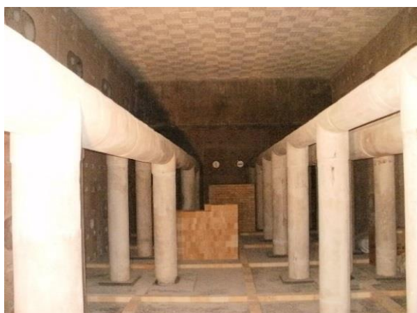
Fig. 1 Inside view of heating furnaces furnace equipped with regenerative burner.
