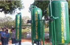
Ensuring a safe and securing living environment through the provision of clean drinking water by the installation of purification equipment
