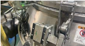
The opening of mixer is equipped with a limiter switch, which prevents people from approaching while the mixer is in operation.
