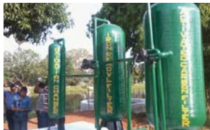
Ensuring a safe and securing living environment through the provision of clean drinking water by the installation of purification equipment
