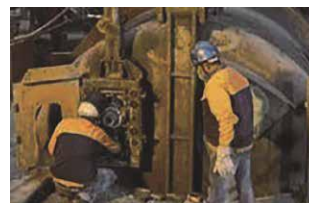
Refractories management at a customer production site
