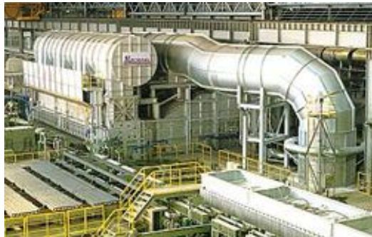
Example of construction work: pusher type billet continuous hot rolling reheating furnace
